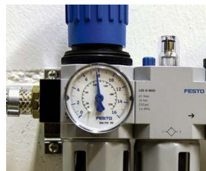
Fig. 13 Deoiler for compressed air
