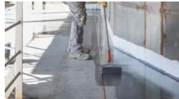
Application of SikaCor® ZP primer with a roller on a steel deck
