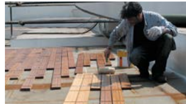
Application of Sika® MultiPrimer Marine with a roller on a teak deck (reverse side)
